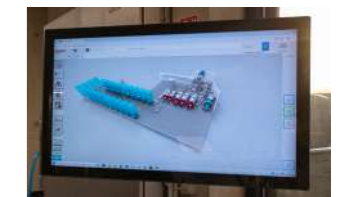
Main screen/remote control consoles
